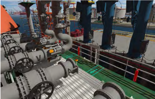
Figure 1. LNG transfer platform in ship-to-shore scenario.
